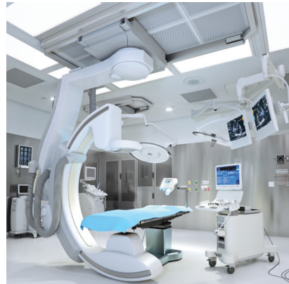
Hybrid Operating Room
