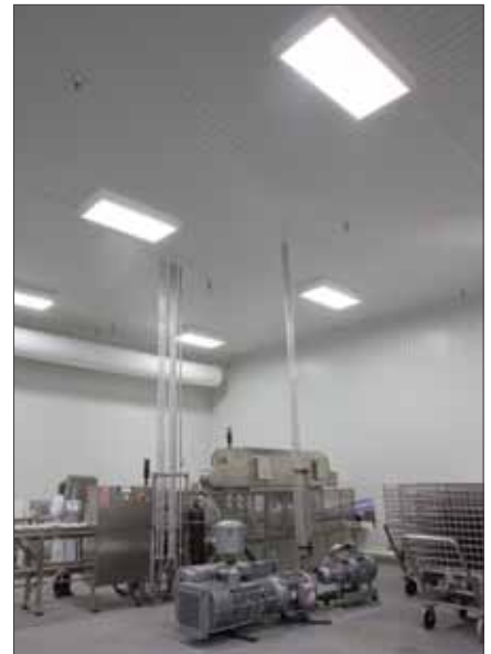
Kenall’s SimpleSeal provides safe lighting for U.S. Pet Nutrition plant in Lyons, GA
